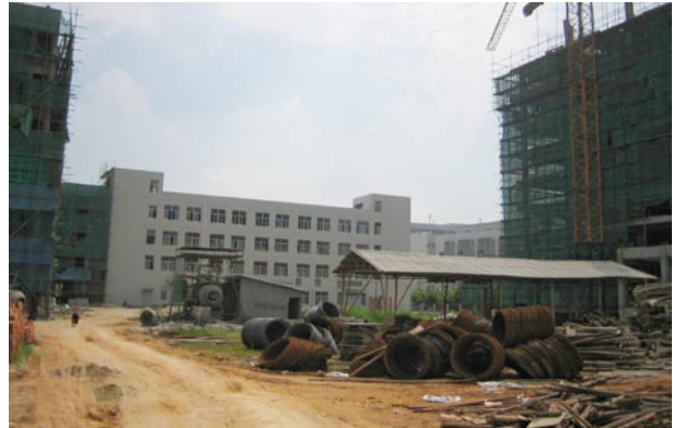
Construction of a new manufacturing facility that will double capacity and be ready in early 2010
